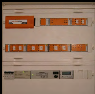
example of a central computer of the Arcos Comfort system
